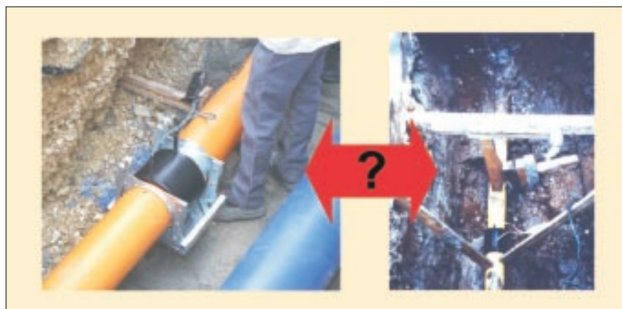
Fig. 3: The use of holders versus conventional, time-consuming methods, which should be avoided in order to achieve good installation quality
